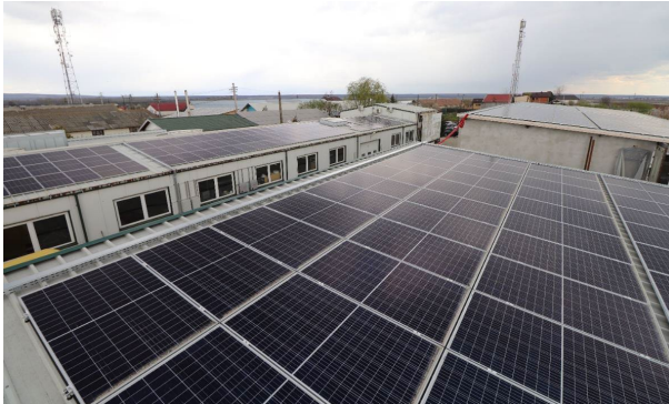
PV Generator 130kWp
