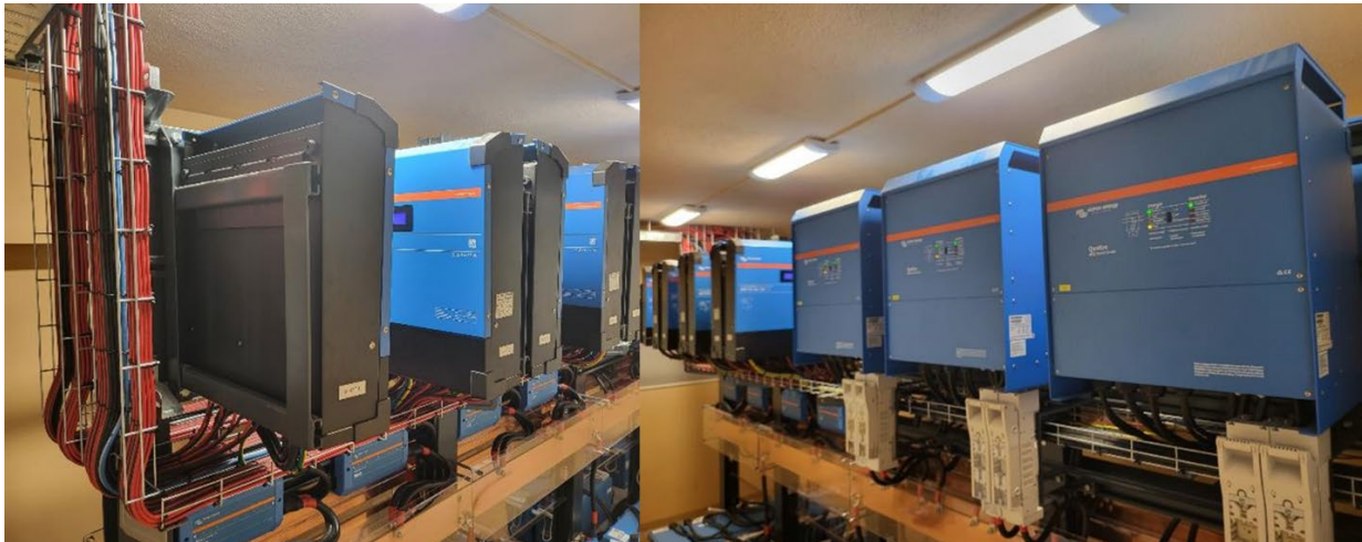
Technical room for Power conversion (90kVA) and storage (LiFePo4 100kWh)
