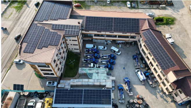
PV Generator 140kWp
